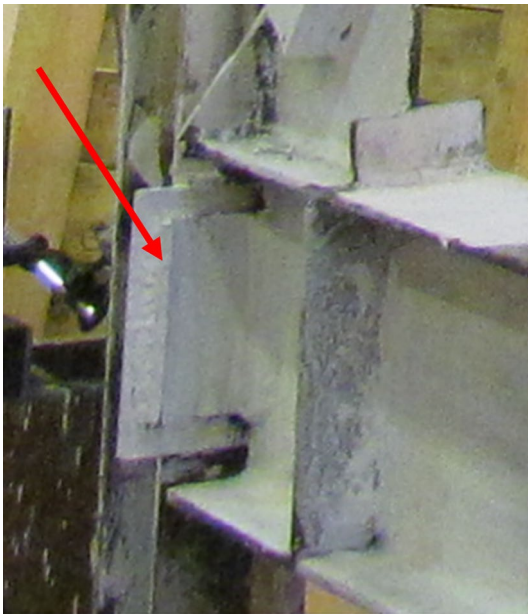
Fig. 10 Using additional plate on the columns flanges to have more flexible web clip angles in Fr.2
